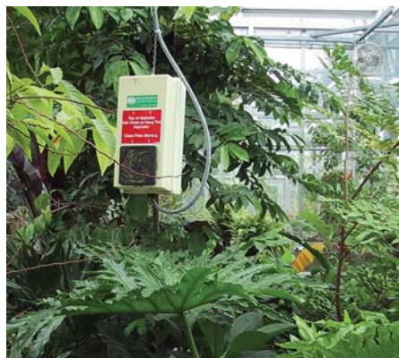
Top right: Environmental controls can determine when the equipment needs to turn on. In this example, the contactor panel is the muscle that tells the equipment to turn on; it's also known as motor starters. The vent control box has small relays to signal the drive unit (motor) to operate. Above: This is an aspirated temperature sensor. It is housed in a solar-guarded box with a fan that pulls air across the sensor. It should be hung at crop level as the temperature higher in the greenhouse can be a lot warmer. It is important to clean the filter monthly to ensure sensor accuracy. (Photos: Wadsworth Control Systems)
