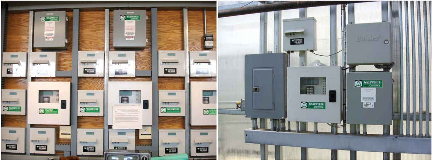
Left: These controls each have their own contactor panel, power pull energy curtain control box and four vent control boxes. This is a complete system. Right: This is an EnviroSTEP control, contactor panel and vent control box at a garden center.
